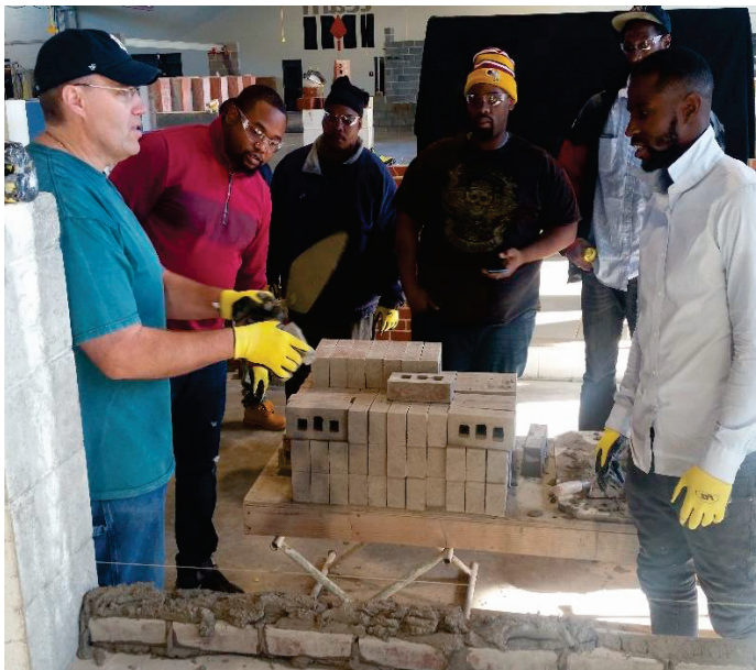
Building Futures students learn about masonry at the union International Masonry Institute
